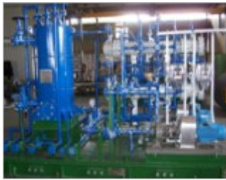
Auxiliaries Skid Packaging Client: Dresser Rand End User: Samir Flare Gas
